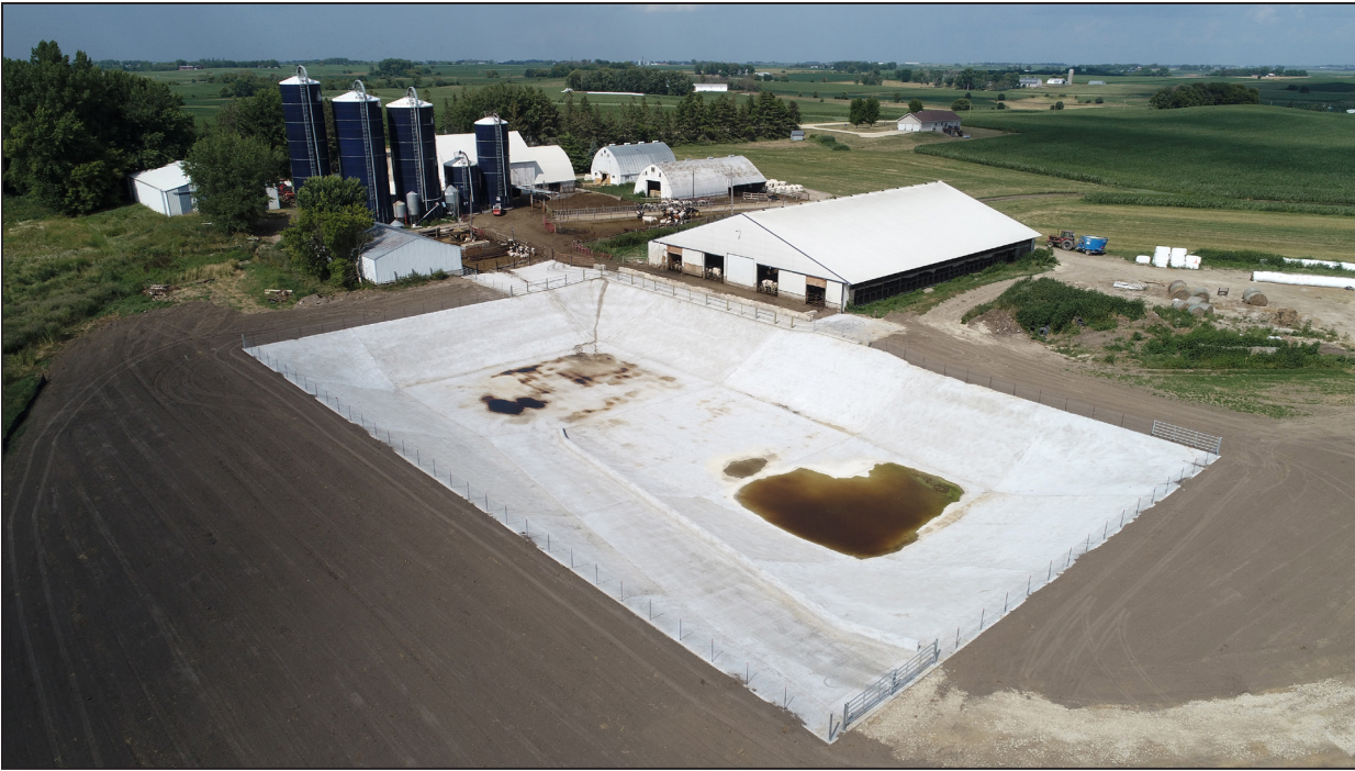
Watershed-Based Implementation Funding supported the feedlot upgrade on Tony Scheffler's Minneola Township dairy farm. The new manure pit has the capacity to hold 14 months of manure, which means Scheffler can apply that nutrient when conditions are right and the plants need it most.
