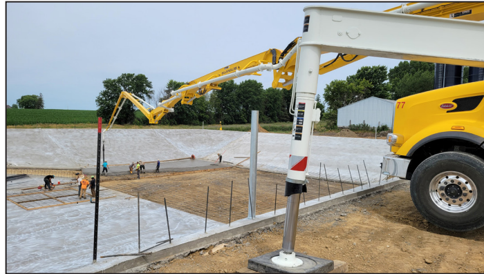
The manure pit was constructed in 2023. It contains runoff, preventing it from entering a creek that flows to the North Fork Zumbro River.
