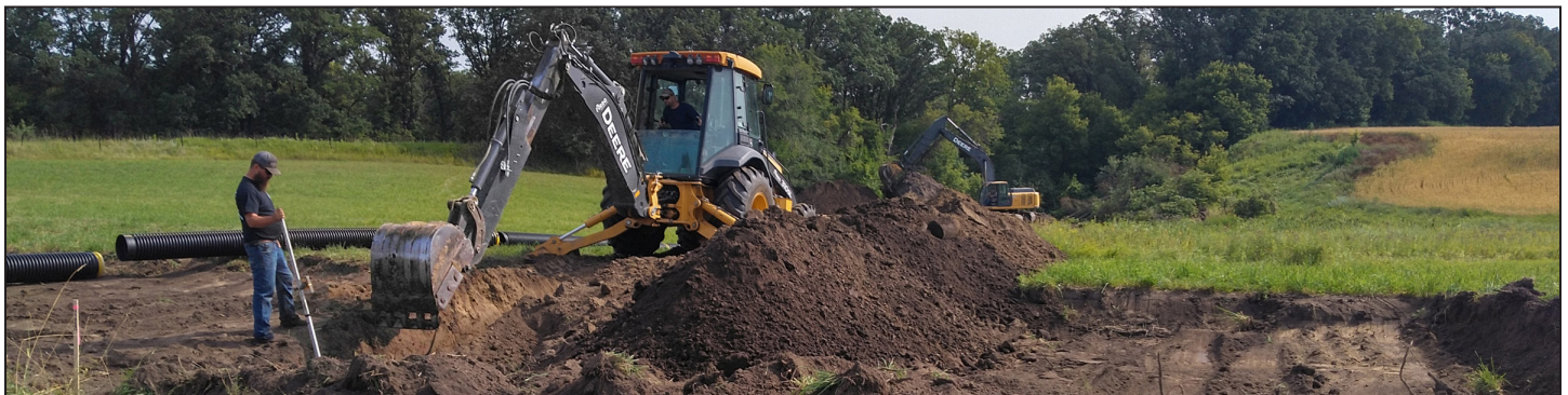
Projects involving North Pod engineering staff included a grade stabilization in Red Lake County. Photo courtesy of Red Lake County SWCD
