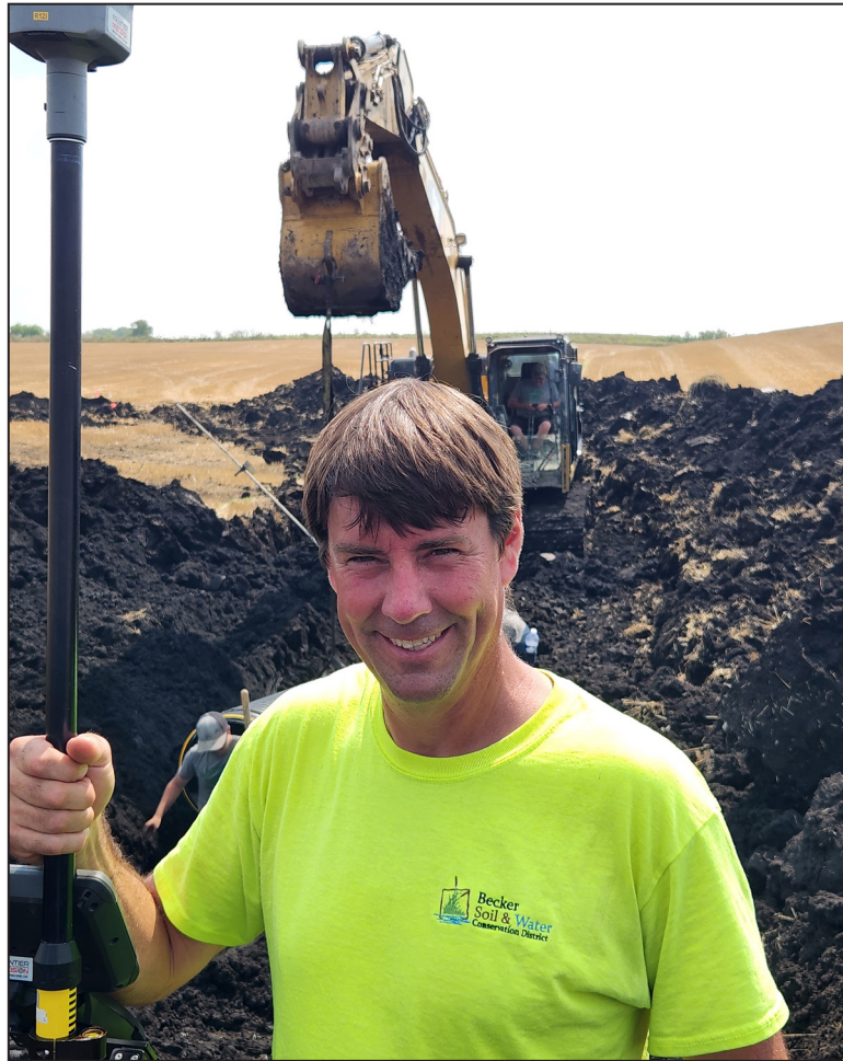
Becker SWCD-based South Pod Engineer Wes Drake staked tile lines and conducted post-installation surveys in August within the West Otter Tail County district where construction of a stabilization structure and water and sediment control basins was underway. Photo courtesy of Wes Drake
